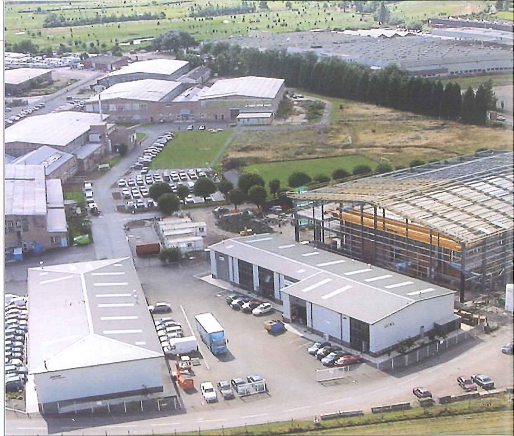
This view, taken in 2001, shows the frame of the new building being erected around the original test department hangar.
